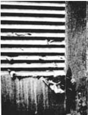
Here, a latex top coat was applied directly over old oil paint, resulting in intercoat peeling. The latex was unable to adhere. If latex is used over oil, an oil-base primer should be applied first. Photo: Mary L. Oehrlein, AIA.
