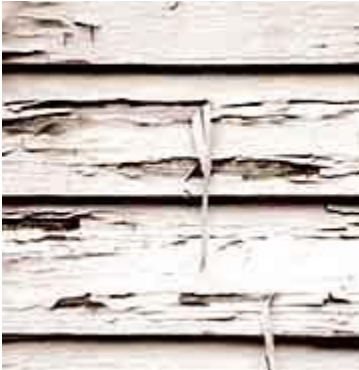
Extensively deteriorated paint needs to be removed to bare wood, then primed and re-painted. Photo: NPS files.
