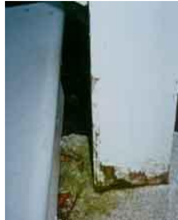
The problem evidenced here by mossy growth and deteriorated wood must be resolved and the wood allowed to dry out before the wood is repainted. Photo: NPS files.
